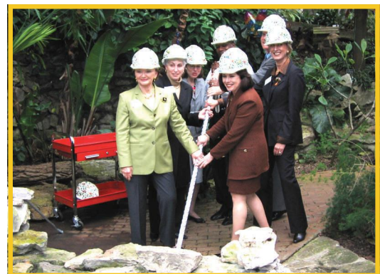
Long time project supporters turn the first stone at the renovation ceremony for the Texas Discovery Gardens
